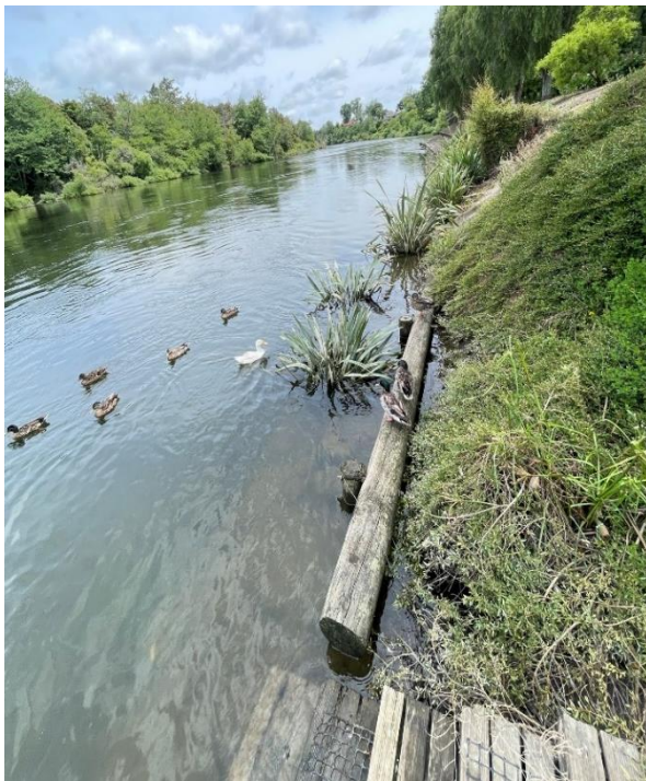
Figure 14. Swarbrick Landing - Jetty during high flow showing difficult egress points if stairs are missed
