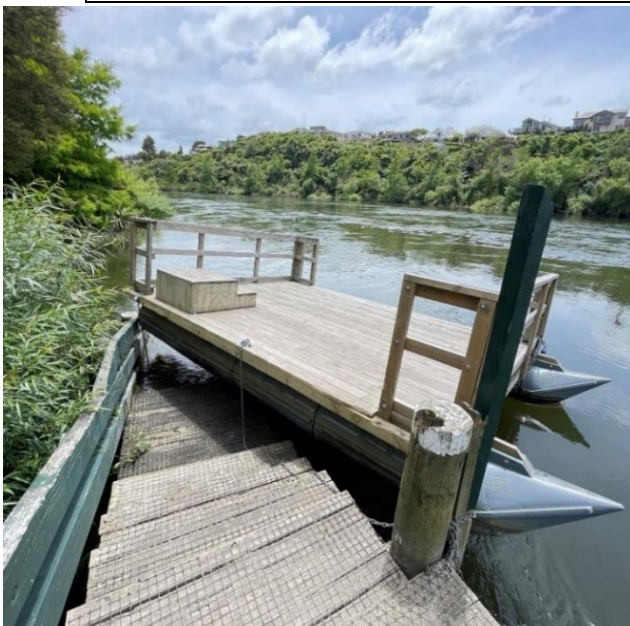
Figure 16. Braithwaite Jetty - Displaced pontoon jetty
