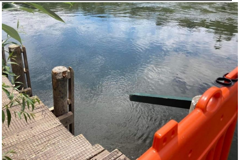
Figure 15. Braithwaite Jetty - Closed site and damage to support beams
