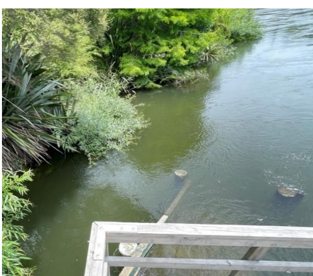
Figure 17. Braithwaite Jetty - Entrapment risk underneath pontoon
